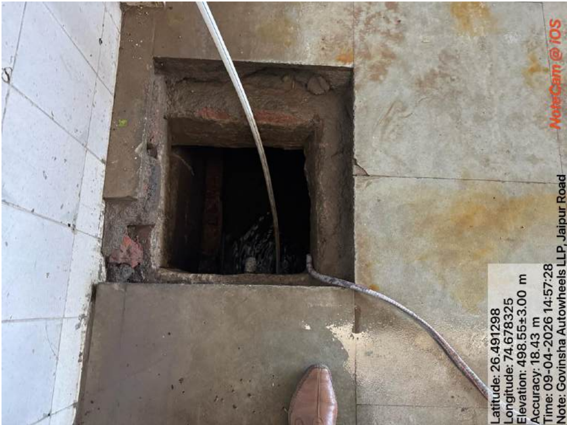
Waste water storage tank
